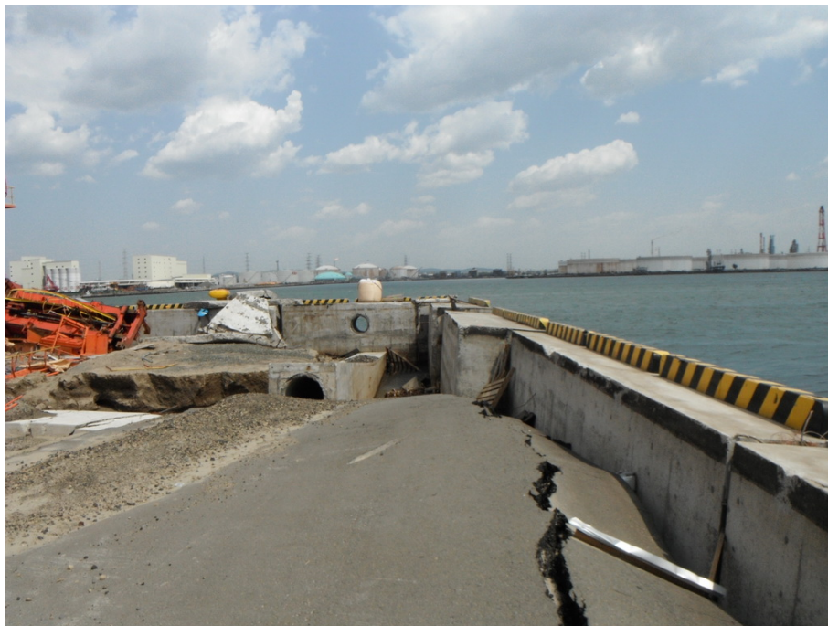
Fig. 6.16 Rotated wharf closure bulkhead at the east end of the Takasago wharf (Percher, 2014)
