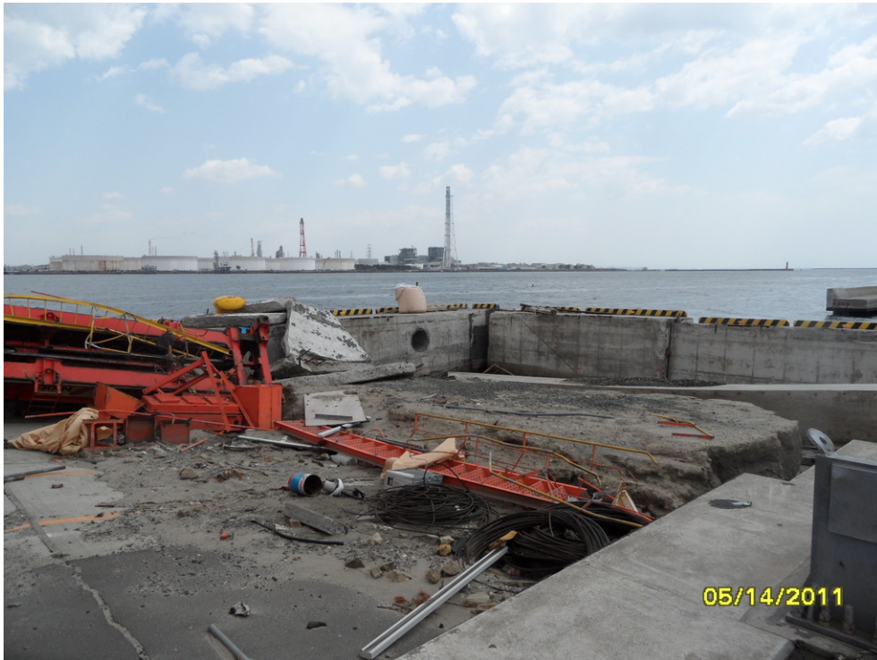
Fig. 6.17 Significant vertical settlement near the east end the Takasago wharf (Percher, 2014)
