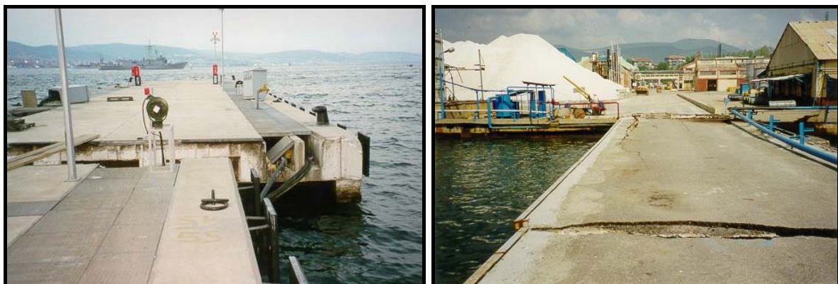
Fig. 6.27 A displaced steel piped jetty in Izmit (left) and a damaged jetty at Gölcük Naval Base (Bilham et al., 2003)
