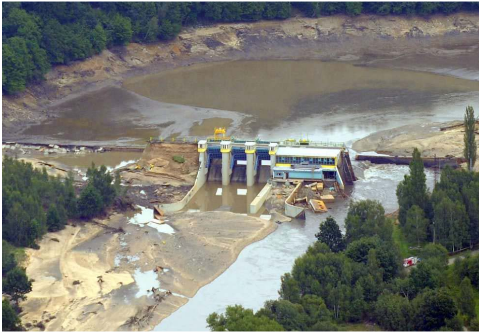
Fig. 3.2 Failure of the Niedow dam in Poland due to flooding (taken from Fry et al., 2012)
