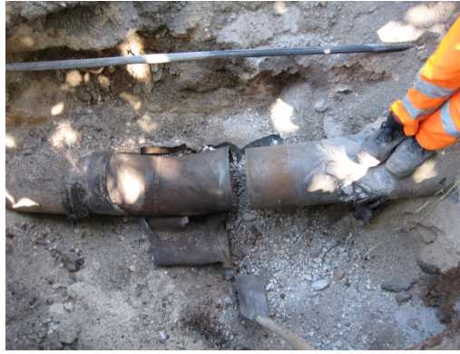
Fig. 5.1 Damage to gas pipes following the L`Aquila earthquake: gas welded joint of a LP steel pipe pulled apart in Paganica (Esposito et al., 2013)
