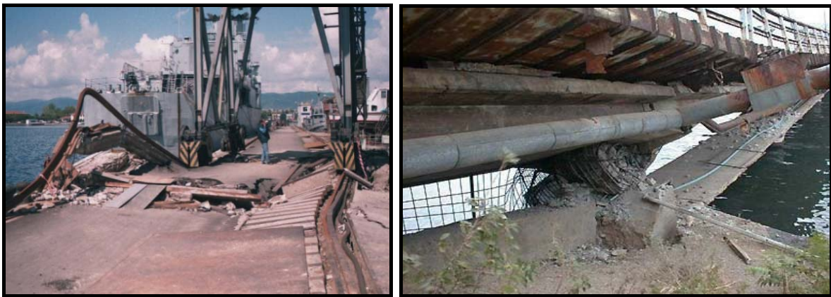
Fig. 6.26 Damage at the navy port in Gölcük (left) and failed column at SEKA port (right)
