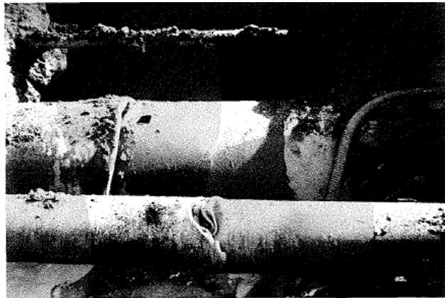
Fig. 5.9 Compression failure of gas and water lines (Lau et al., 1995)
