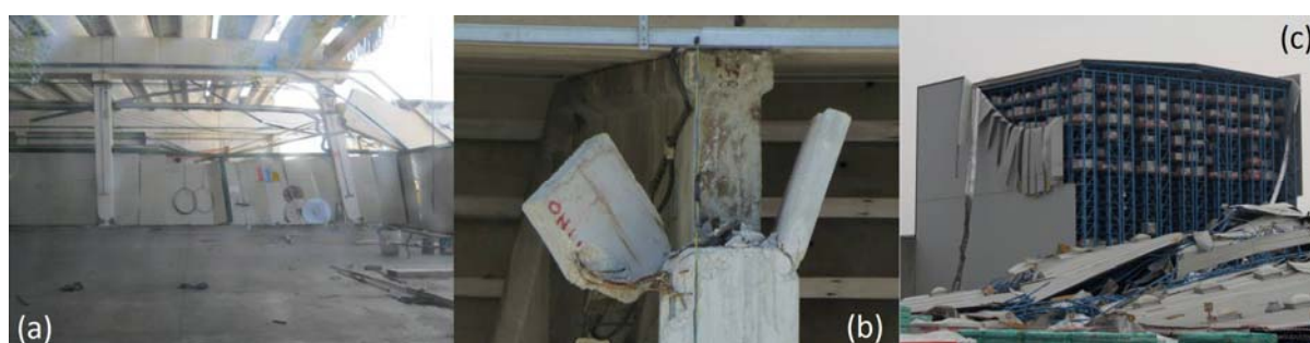
Fig. 7.13 Observed damage to industrial buildings (taken from Liberatore et al. (2013))
