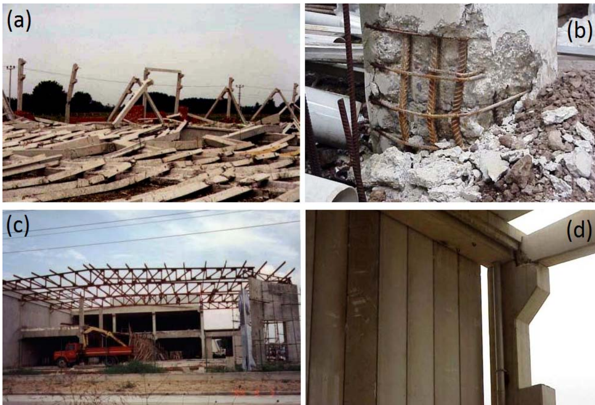
Fig. 7.4 Precast structures in the same industrial zone under different construction stages and corresponding damage levels (taken from Saatçioğlu et al. (2001))
