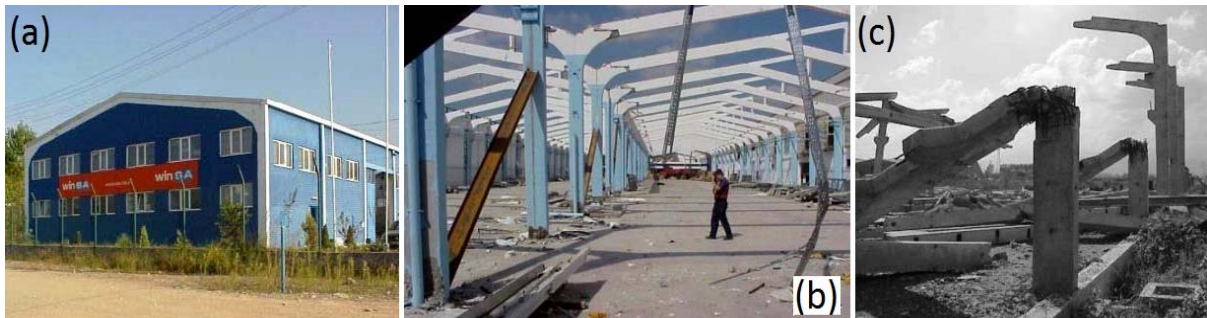
Fig. 7.3 Precast Industrial buildings sustained various degrees of structural damage (taken from Saatçioğlu et al., 2001)
