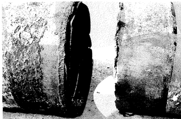
Fig. 5.10 Tension failure of gas line (Lau et al., 1995)
