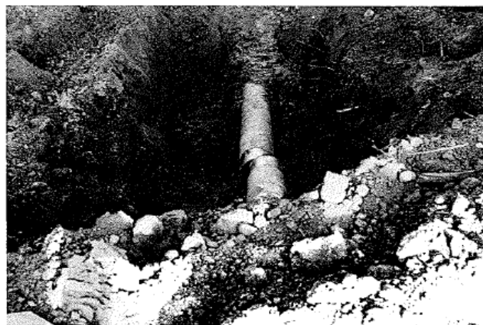
Fig. 5.8 Shear failure of gas line (Lau et al., 1995)
