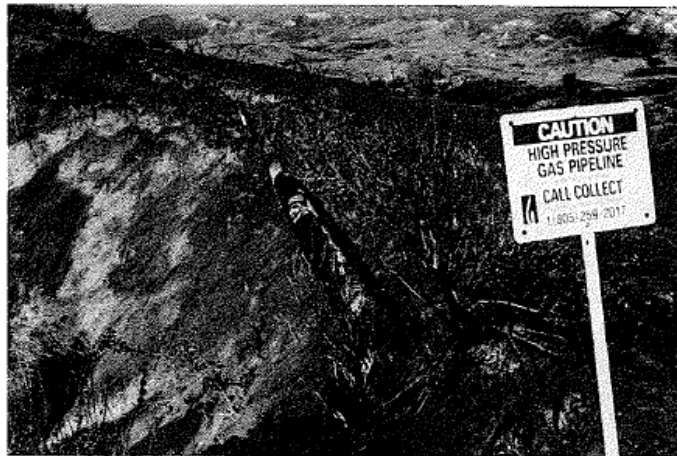
Fig. 5.7 Buried gas line exposed by landslide (Lau et al., 1995)
