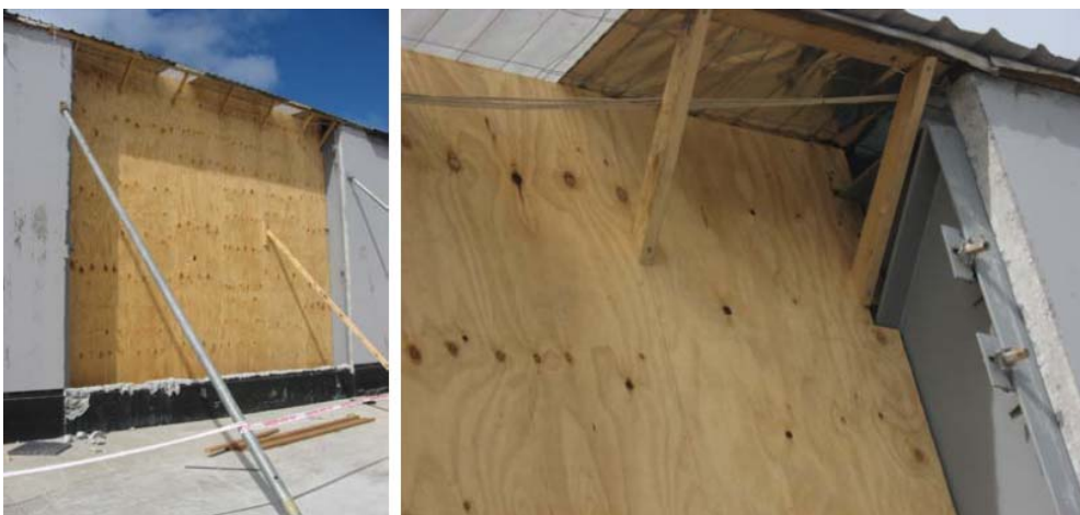
Fig. 7.12 Panel collapse due to steel frame connection failure (taken from Marshall and Gould (2012))
