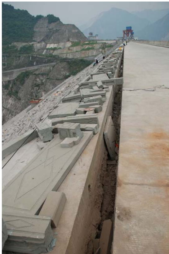
Fig. 3.1 Fracture at the Zipingpu dam's crown (taken from Lekkas, 2008)
