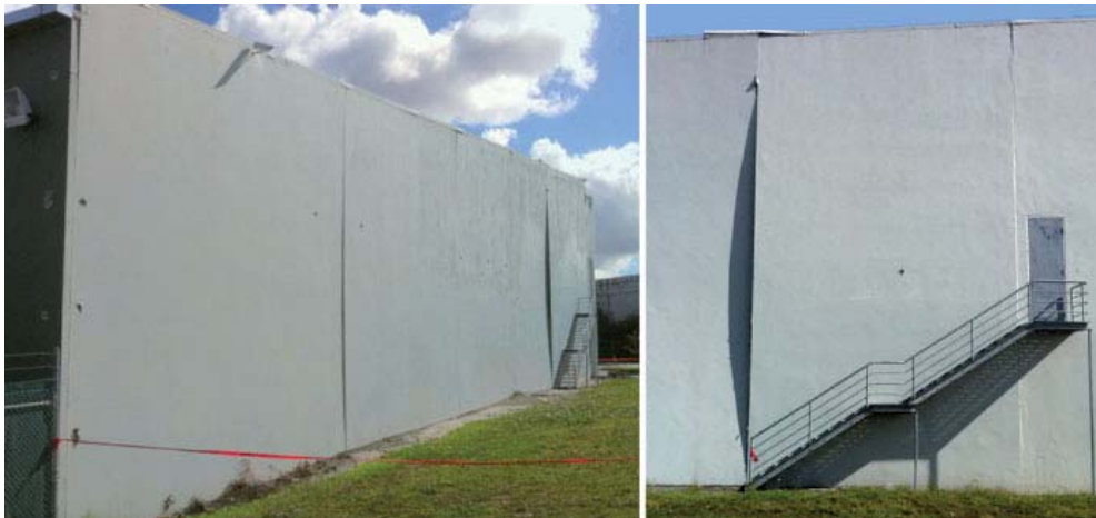
Fig. 7.11 Out-of-plane buckling of concrete wall panels (taken from Henry and Ingham (2011))
