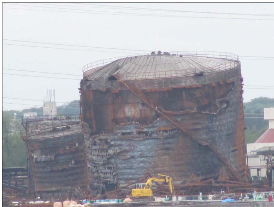
Fig. 2.11 Burned hydrocarbon tank at the JX Sendai refinery (TCLEE, 2012)
