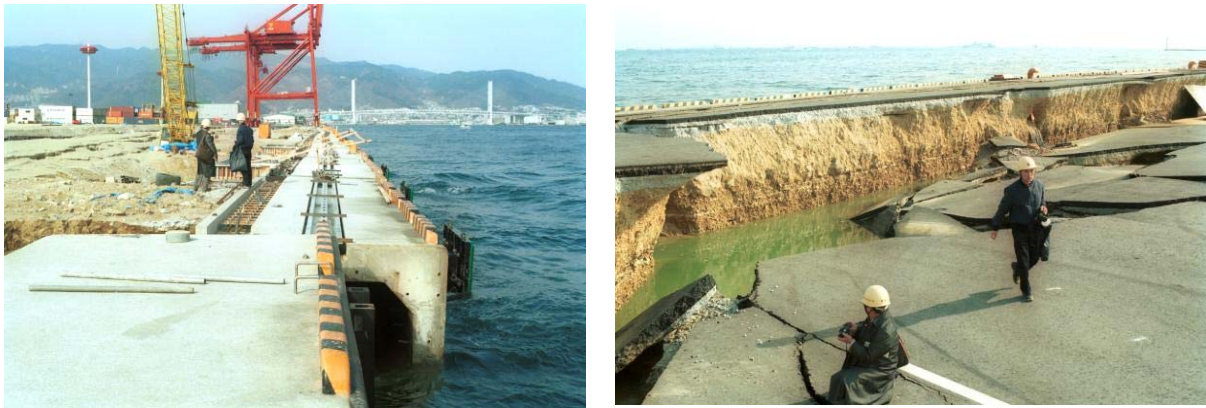
Fig. 6.4 Seaward displacement and tilting of quay-walls
