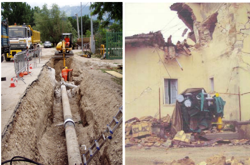
Fig. 5.3 Damage to stations: repairs to the input/output network of Onna M/R and inclusion of stop-system (left); RG housed in a masonry kiosk closed to building and damaged following the earthquake (right) (Photos courtesy of ENEL Rete Gas)
