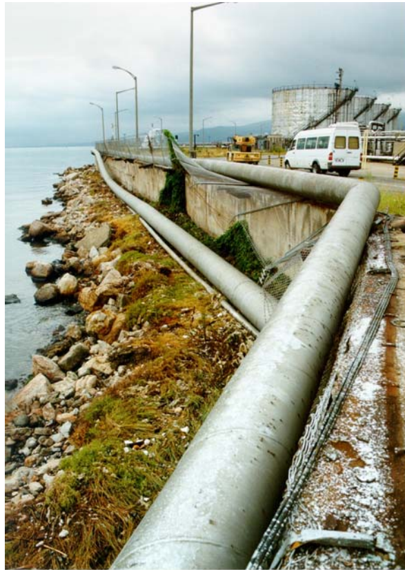
Fig. 4.1 The ground-supported unseated crude oil unloading pipeline fell from the supports at TUPRAS refinery due to inertial effects (Courtesy of TUPRAS (2000))
