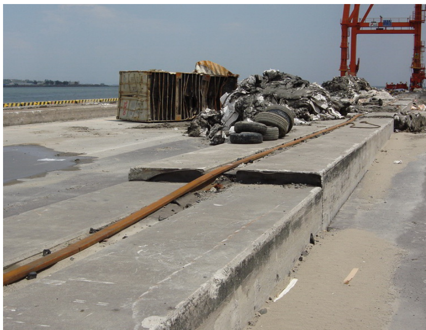
Fig. 6.19 Differential vertical movements of the crane rail girders and settlement of fill surface (Percher, 2014)
