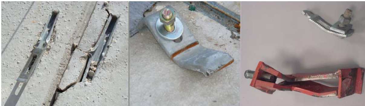
Fig. 7.8 Damage to connections and fastenings (Toniolo and Colombo, 2012)
