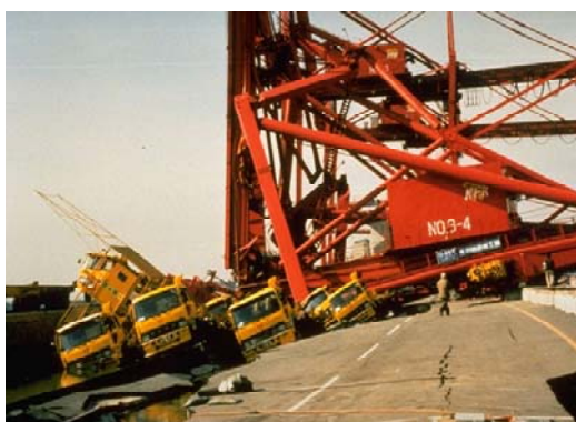
Fig. 6.9 Crane damage due to deformation of foundation soil
