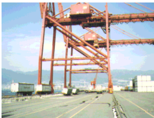
Fig. 6.7 Seaward lateral movement of rail foundation and differential settlement of rails (Rokko Island)
