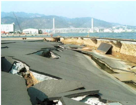
Fig. 6.2 Extremely extensive damage to apron pavements
