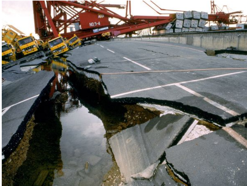
Fig. 6.6 Damage to a quay-wall at the port of Kobe (Nozu et al., 2004)
