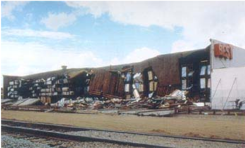
Fig. 7.1 Collapse of roof and wall elements of an old tilt-up building (Photo by G. Sakkestad 2 )
