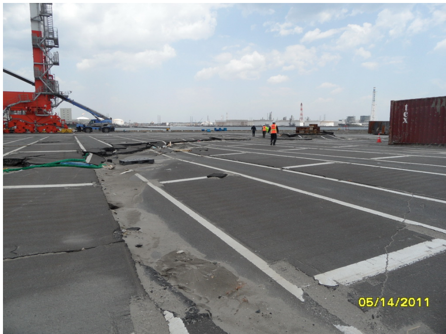
Fig. 6.15 Lateral spreading in the backlands along the original shoreline (Percher, 2014)
