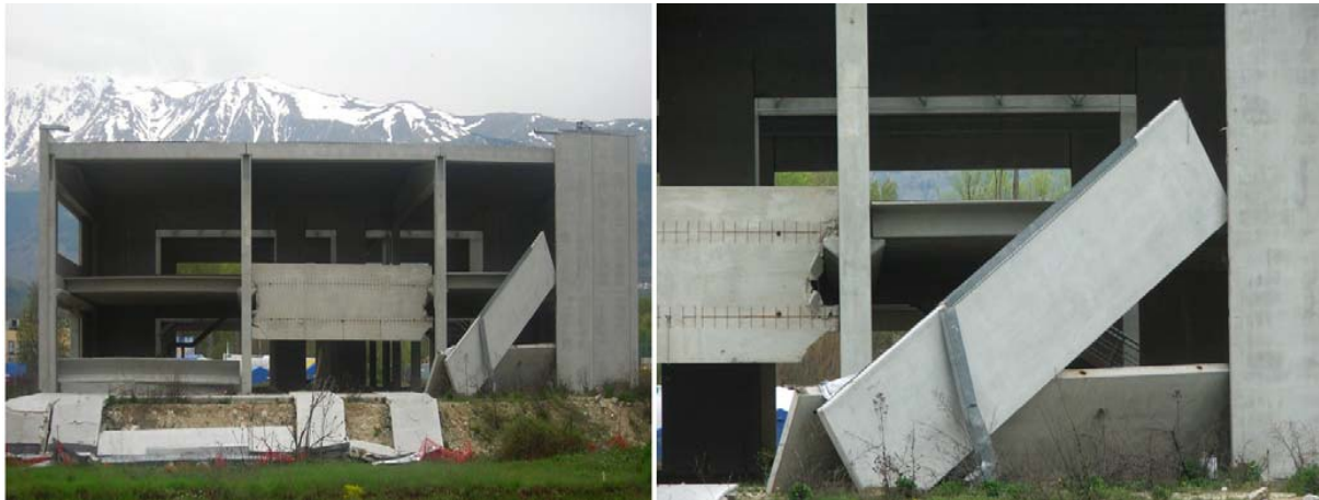
Fig. 7.9 Collapse of precast wall panels (Di Sarno et al., 2011)
