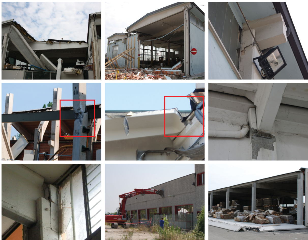
Fig. 2.6 Damage following the first 2012 Emilia earthquake
